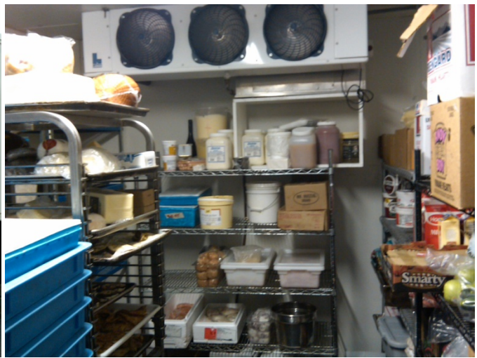
Interior of Walk-in (Bluezone behind Evaporator)
